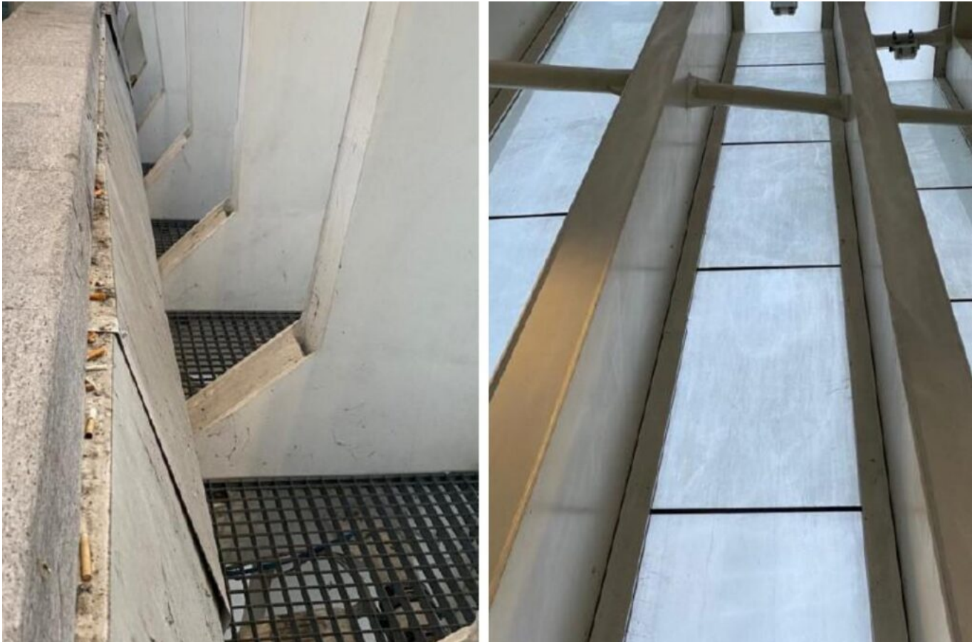
a) Joint between parapet and metal ribs at the height of the boarding sidewalk. b) A section of the ascending glazing with the usual deposit of dust and smog (photo credits Augusto Giuffredi).
